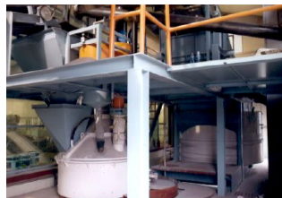
Main mixer, face mixer and platform: Aggregate, cement and water are mixed in Mixer
