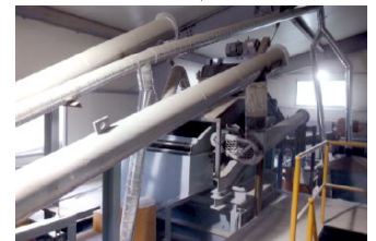
Screw conveyor conveying cement to Mixer
